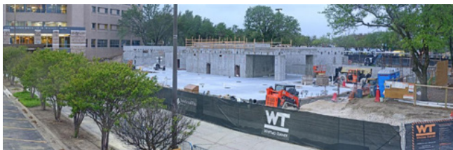
Construction on the new radiation oncology facility at the Baylor Scott & White Vasicek Cancer Center
